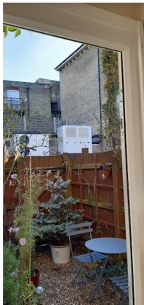
Figure 4: View of the compressor units from our kitchen door.
