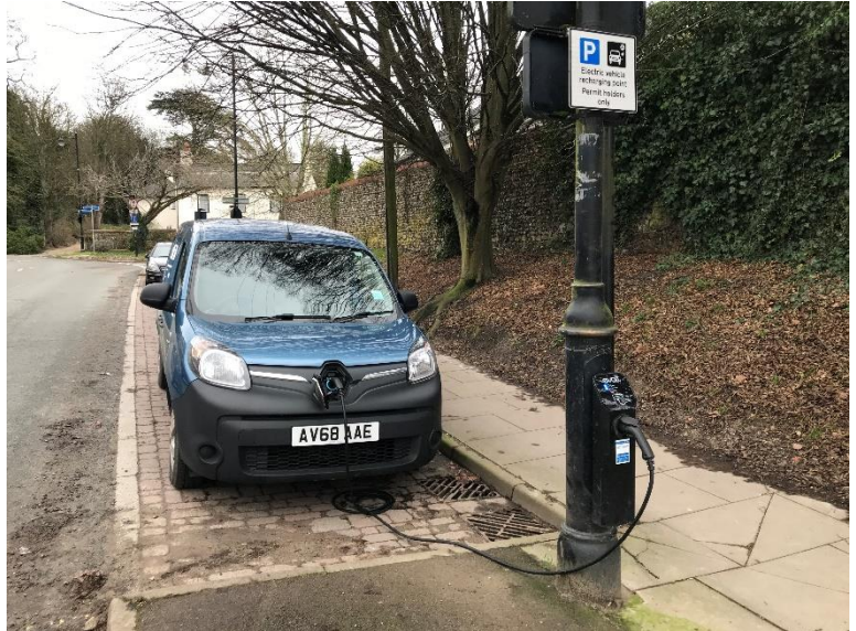
Figure 1: Lamppost EV charger in Bury St Edmunds
